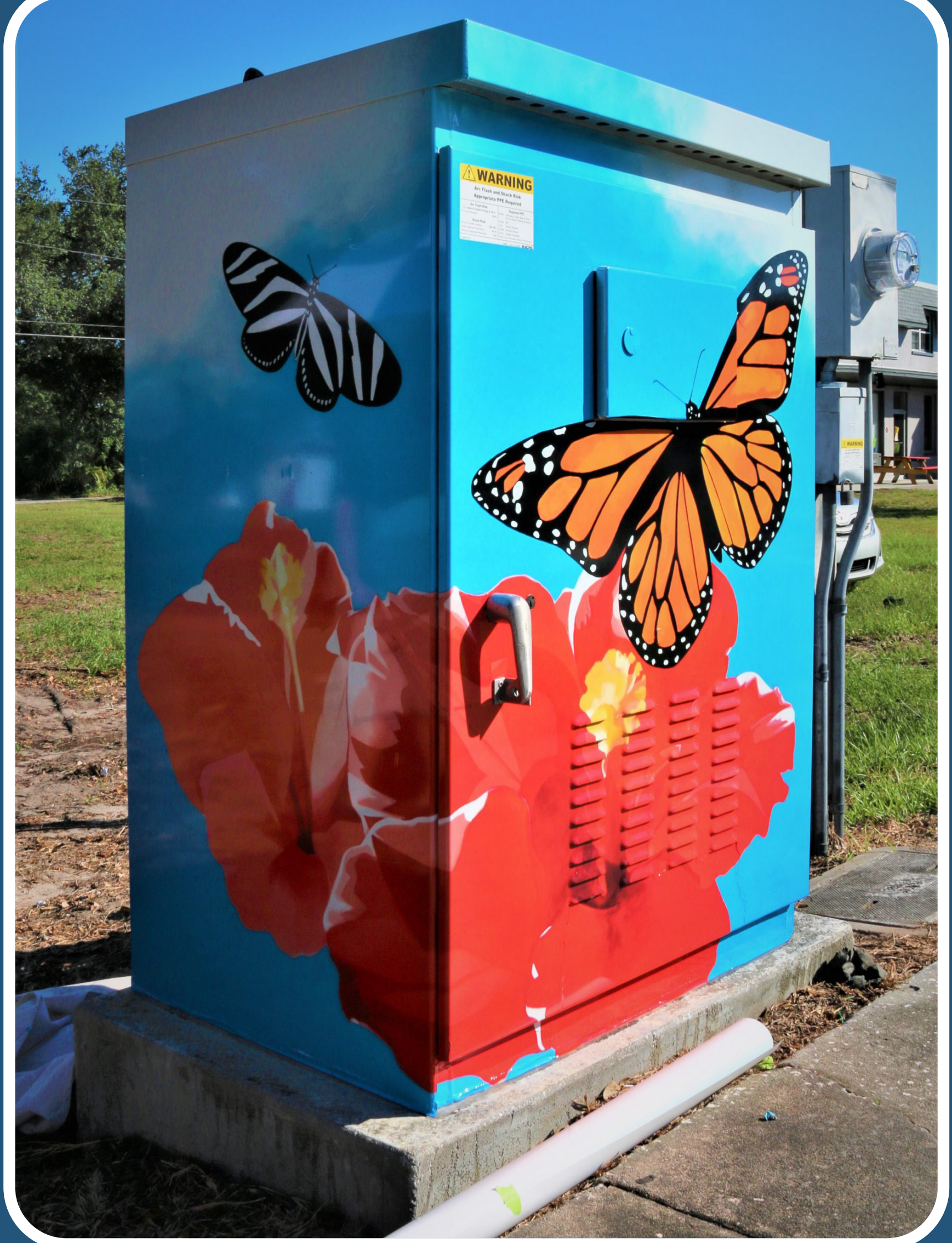
SIGNAL CABINET WRAP
